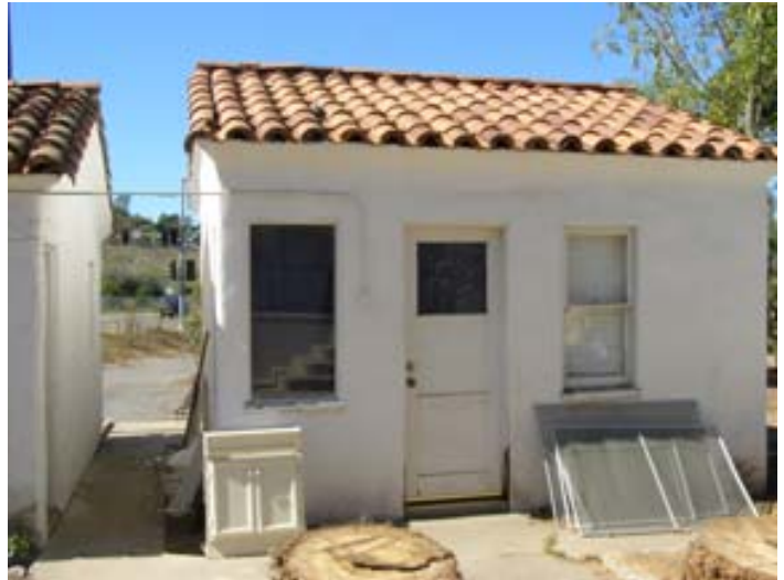
This building is the guest house behind the main house, next to the garage. As part of the construction by the City of Vista, the guest house will be converted to disabled accessible rest-rooms.
